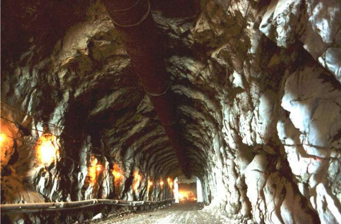
Figure 1.10: An example of poor blasting in a tunnel.
